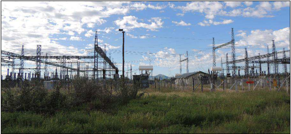
Figure 56 | Photographs depicting the Osona substation sense of place
