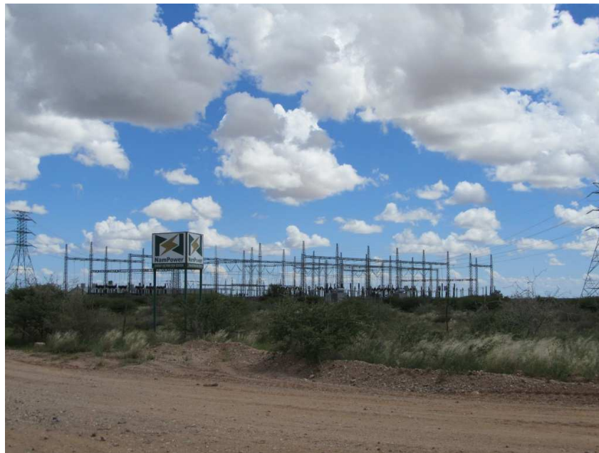
Figure 63 | NamPower's Hardap sub-station
